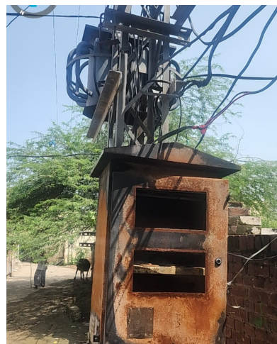
(c) Burnt, empty transformer meter box, August 2026.
